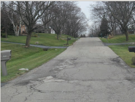
Hoit Tower shows wear before the road paving project began.
