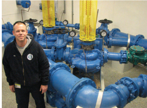
Water Division foreman Ken Brown in the Westbourne Water Pumping Station.
