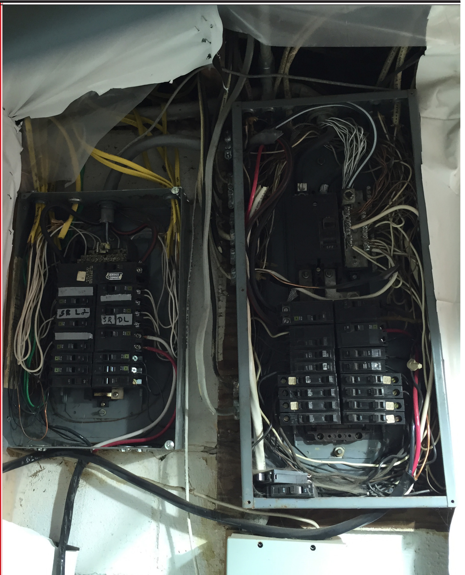
- An overloaded electrical panel.
