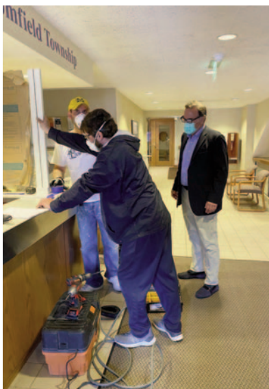
Treasurer Brian Kepes watched as plastic shields were installed at counters in Township Hall.
