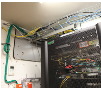
911 equipment is wired in an attic.
