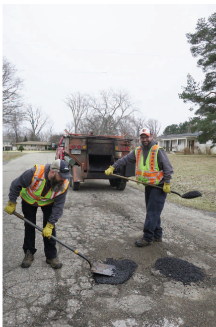
Road Division workers Jason Simpson, left, and Jeff Krauskopf fill potholes in a subdivision.
