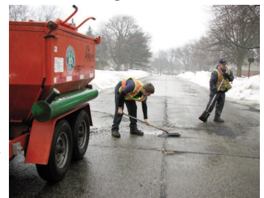
Township crews fill potholes all year long.
